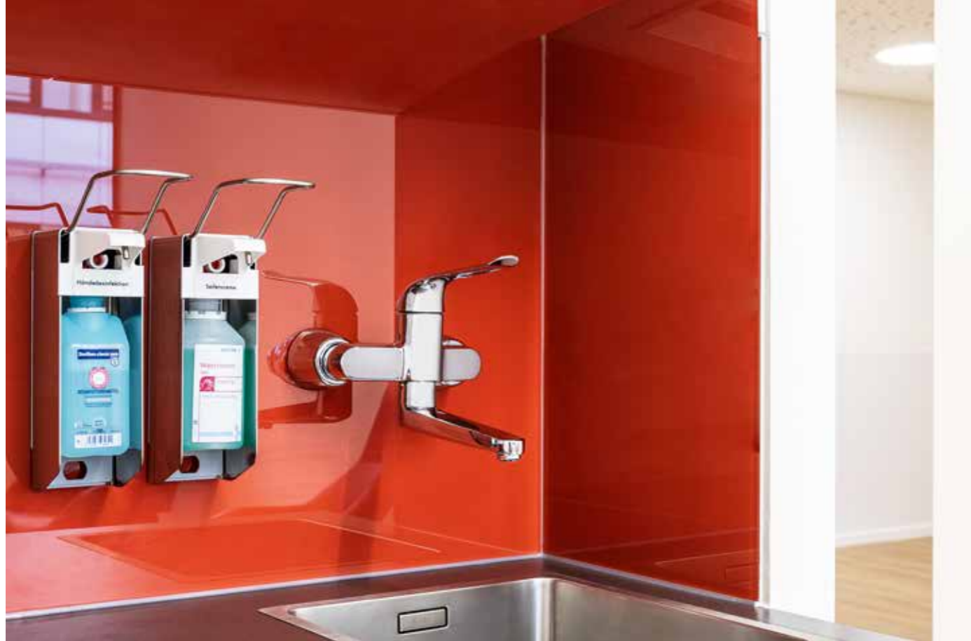
In patient treatment rooms, GROHE Euroeco special safety mixers have been specified; all the functions can be effortlessly controlled by the clinician's elbow – minimizing the risk of germ transmission and maximizing hygiene.
